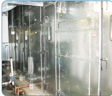
Assembled 38,000 cfm Ventrol AHU that was brought into a tight quartered equipment room through a 60-inch x 60-inch square opening.
